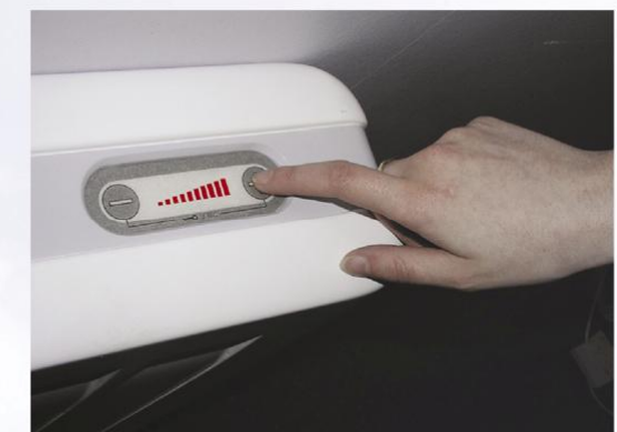
Simple heating controls for residents.
